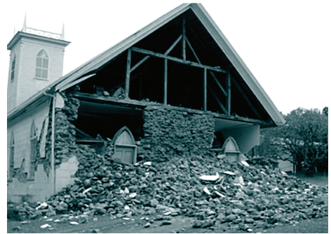
Kalahikiola Congregational Church in Kapa'au, after the October 15, 2006 Magnitude-6.7 earthquake. Photo courtesy USGS.
