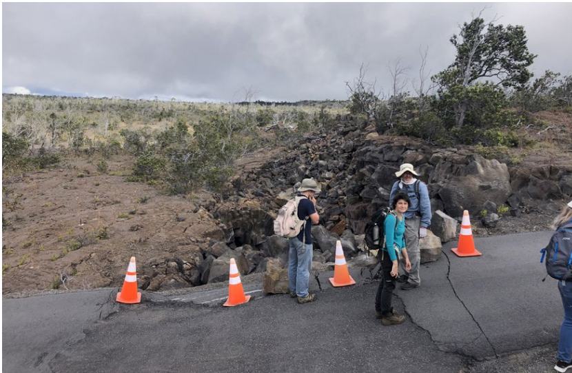
Figure 6. Road damage from surface rupture of the Kulanao'kuaiki fault in 2018.
