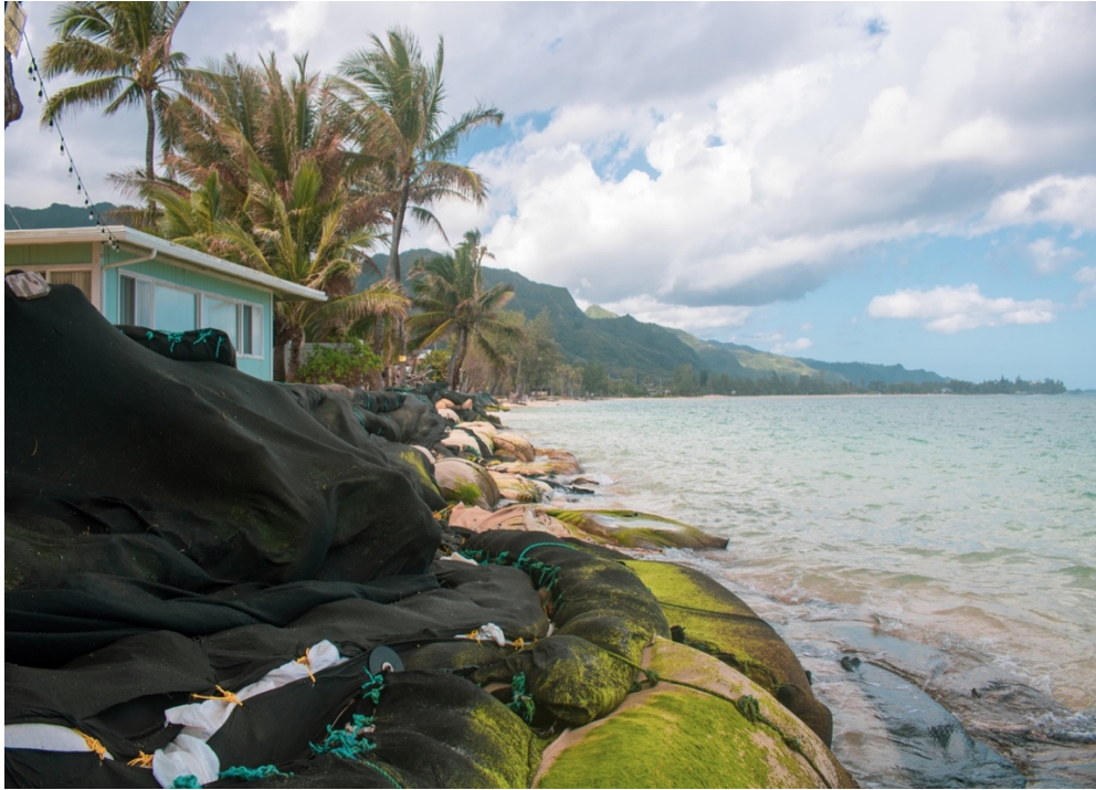
Figure 1. Hardening to protect backshore assets has resulted in widespread beach loss in Hawai'i. Photo of Ko'olauloa shoreline in March 2020 by Kammie Tavares.
